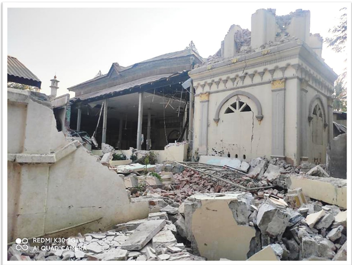
The Kan Oo Mosque in Kyaukse Township, Mandalay Region, after collapsing in the March 2025 earthquake. © BHRN, 2025
