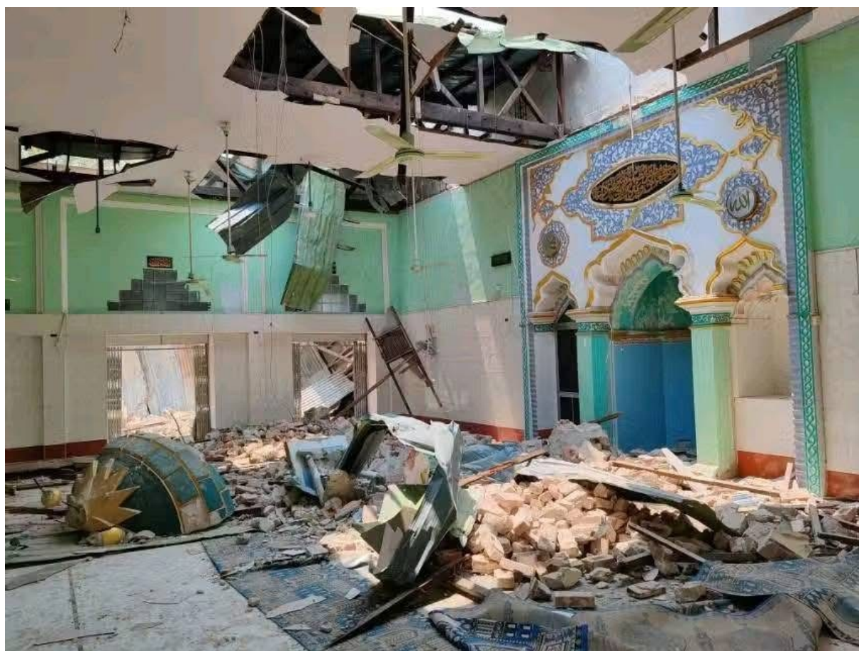
The Ywamonthar Mosque in Ywamonthar village, Tharzi Township, Mandalay Region, after collapsing in the March 2025 earthquake. © BHRN, 2025.
