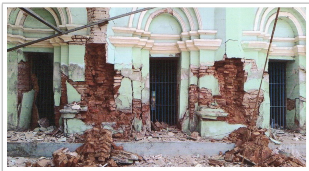
The West Mosque in Taung Myo, Pyigyidagun Township, Mandalay Region, after collapsing in the March 2025 earthquake. © BHRN, 2025.
