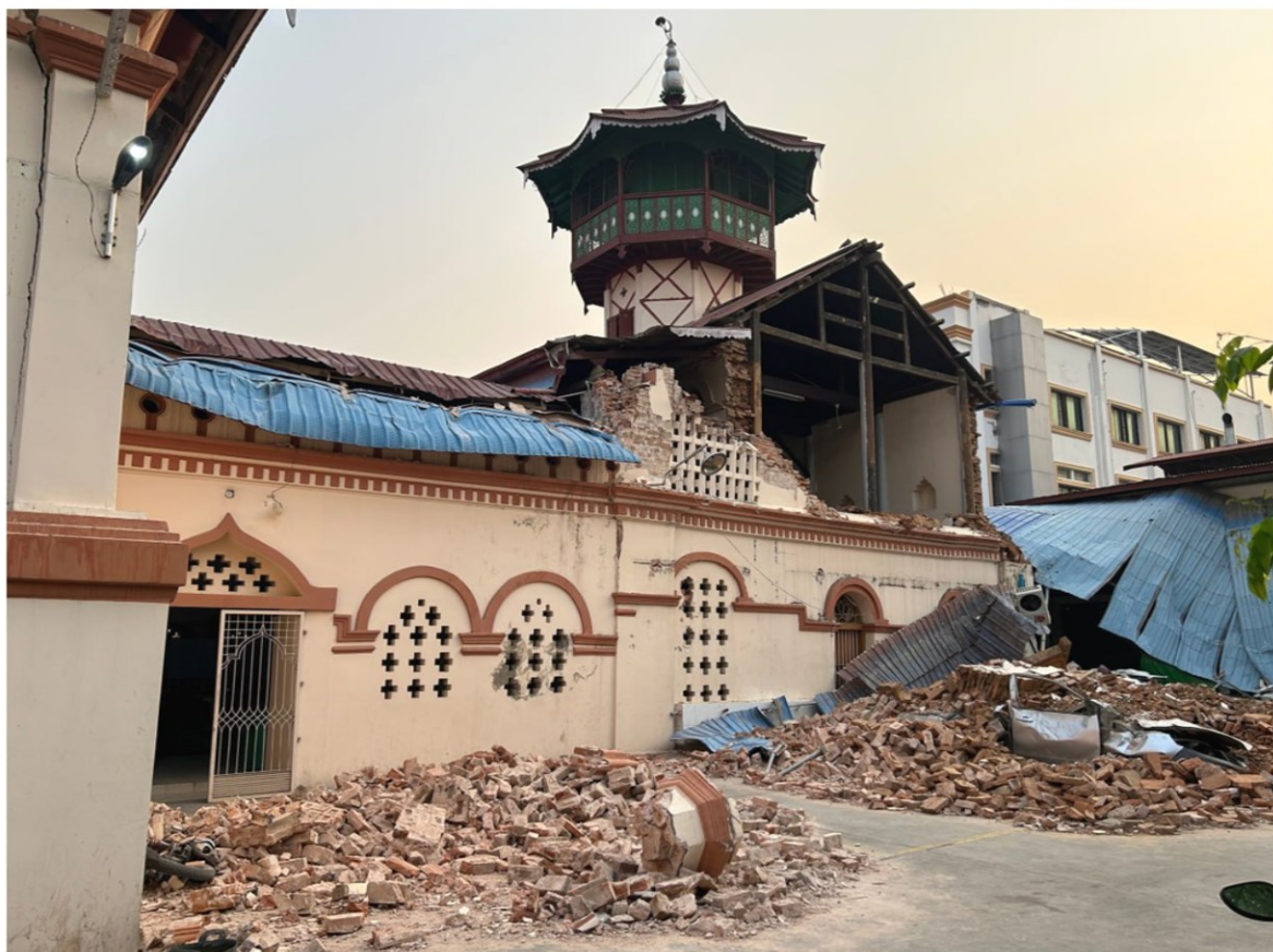
The Panthay Mosque in Maha Aung Myay Township, Mandalay Region, originally built in 1868, after sustaining damage in the 2025 earthquake. © BHRN, 2025.
