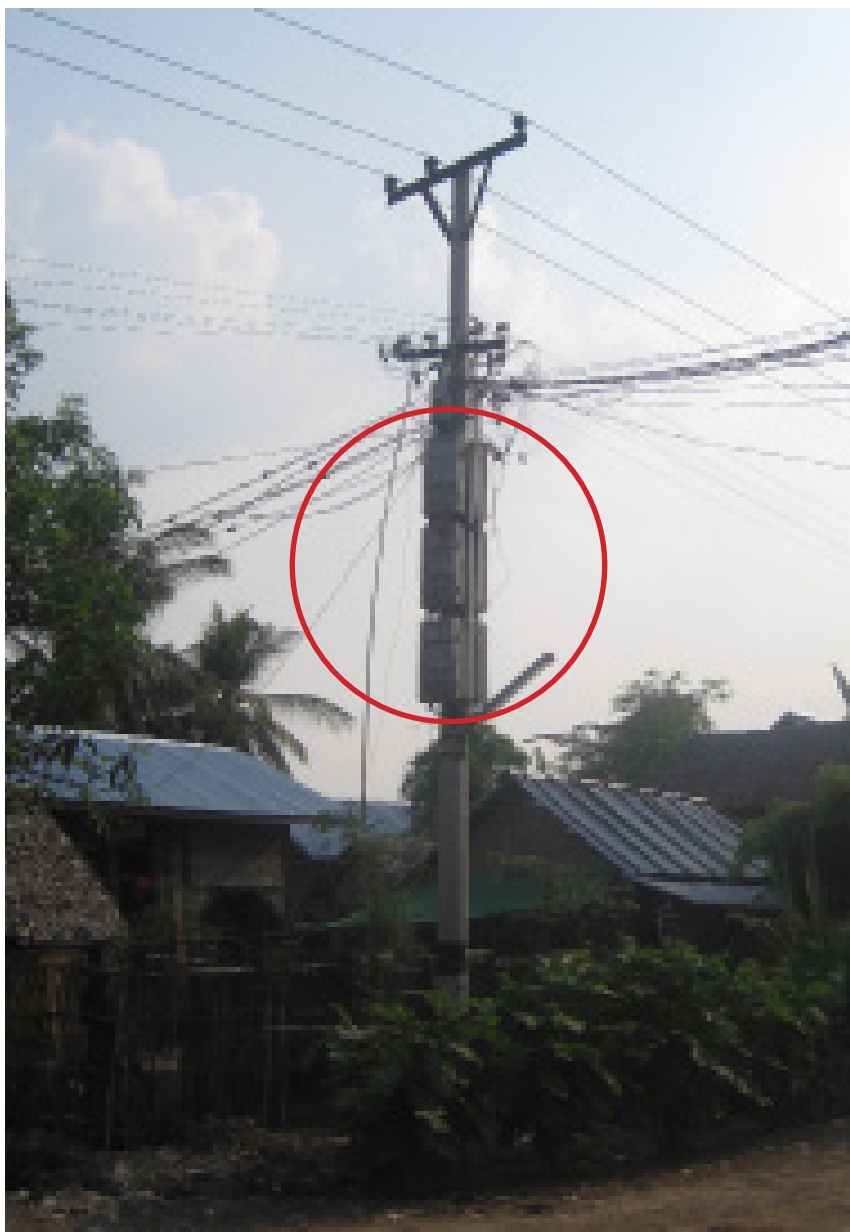
Digital meter on electricity pole
