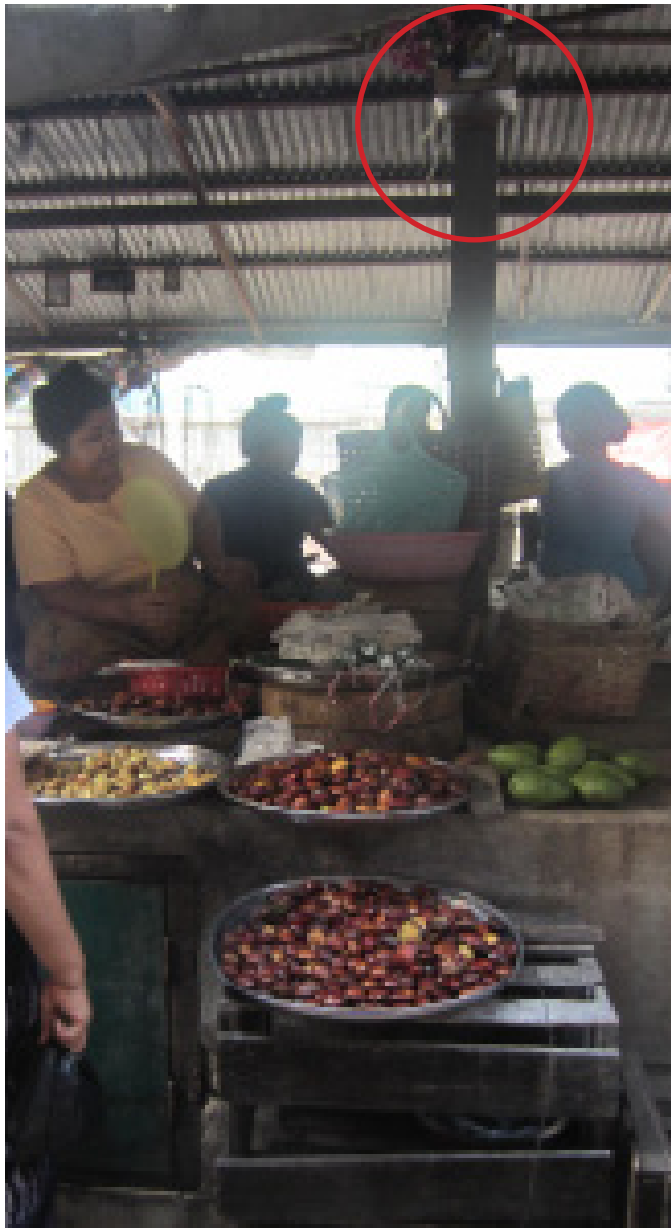
Electricity connection in markets
