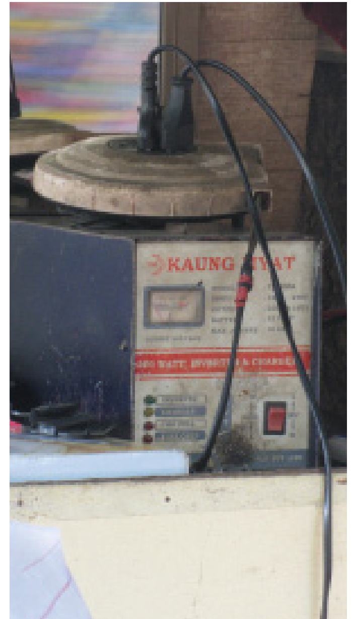
Battery system at Myo's shop
